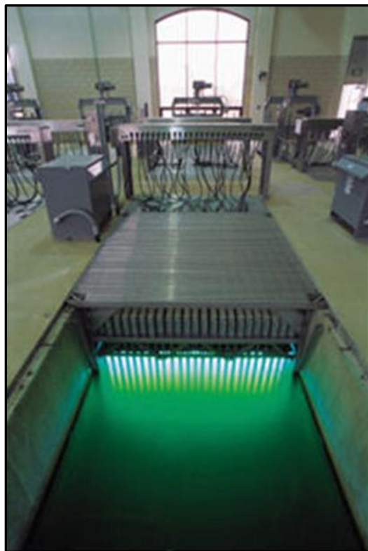
Example of wastewater ultra violet light disinfection. Picture courtesy of Sheldon Primus, Utility Compliance Inc.
